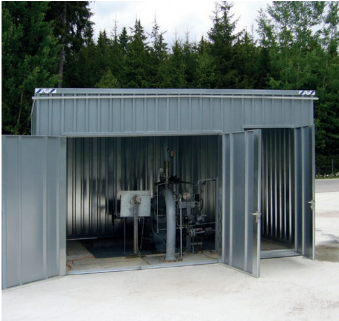
Gas pump housing
